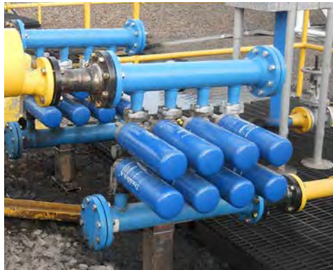
Single-pass Bulk Fuel Filtration System
